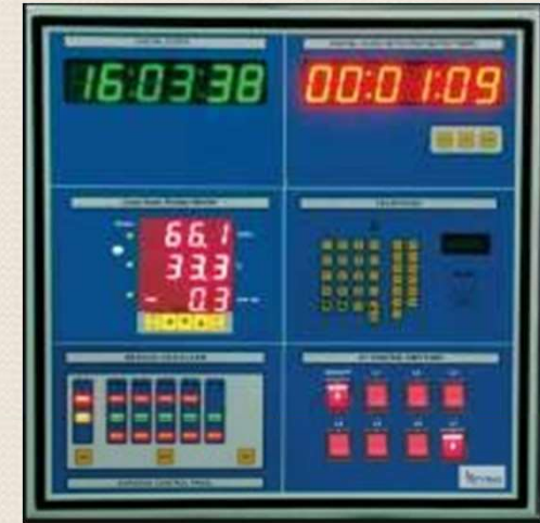
S. Control Panel
