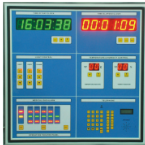
S. Control Panel
